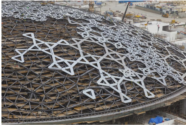
Figure 4.10 – A picture of the dome under construction showing the pattern at the base of each layer, as well as the differences between layers (source http://www.grupo-sanjose.com/ ).
